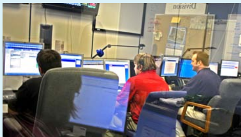
An inside look at MTM's state of the art 24x7x365 Network Operations Center in Wilmington, DE.
